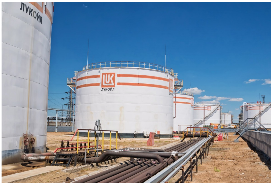
Tank farm for storage of petroleum products in Volgograd, Russia
