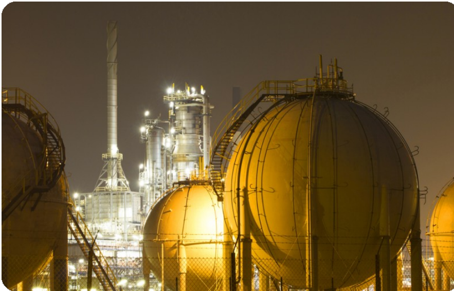
Gas storage tank
