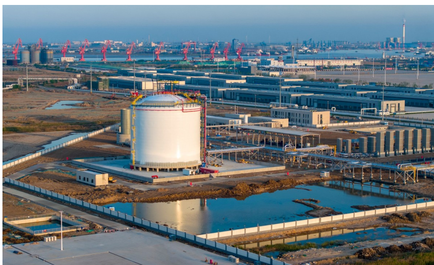
Construction is underway on the LNG storage and distribution station in China's Lianyungang City
