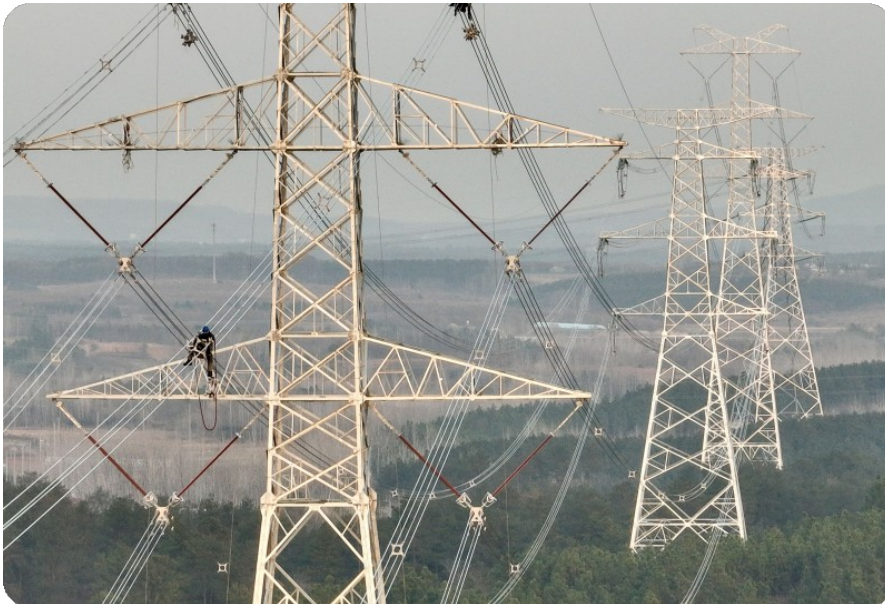
The 136.8km Xiangjian-Ludao 500-kV power transmission line in China's Anhui Province
