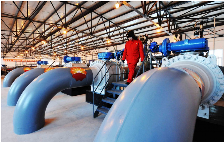
A worker inspects oil pipeline equipment in northeast China
