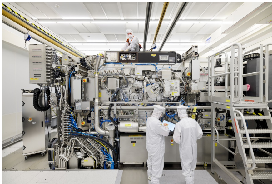
An ASML 'cleanroom' - an ultraclean environment where the company assembles EUV and DUV lithography systems
