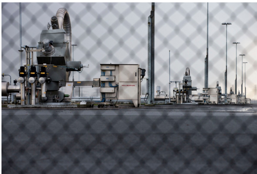
A gas extraction plant in the north of the Netherlands
