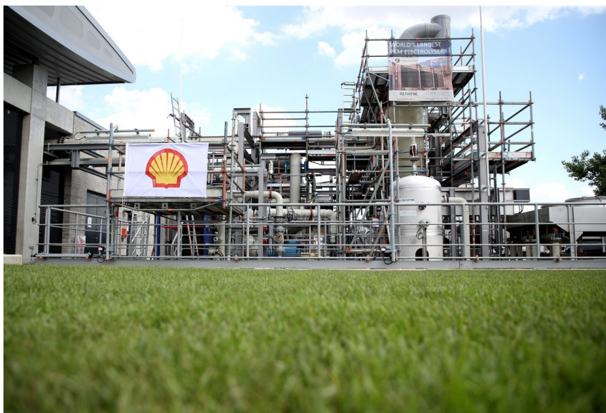
A hydrogen production plant of Shell in Wesseling, Germany
