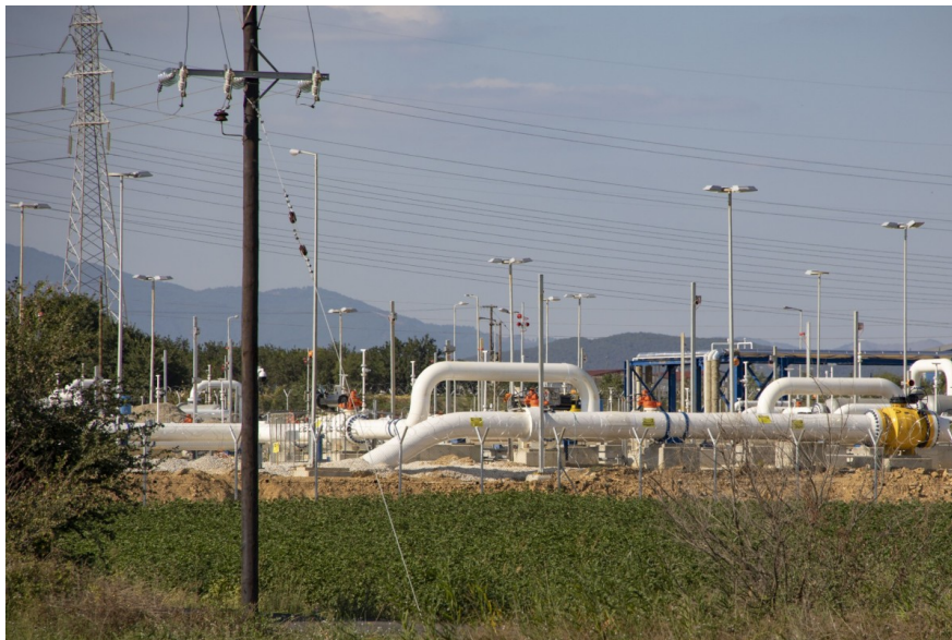
A natural gas pipeline in Komotini, Greece
