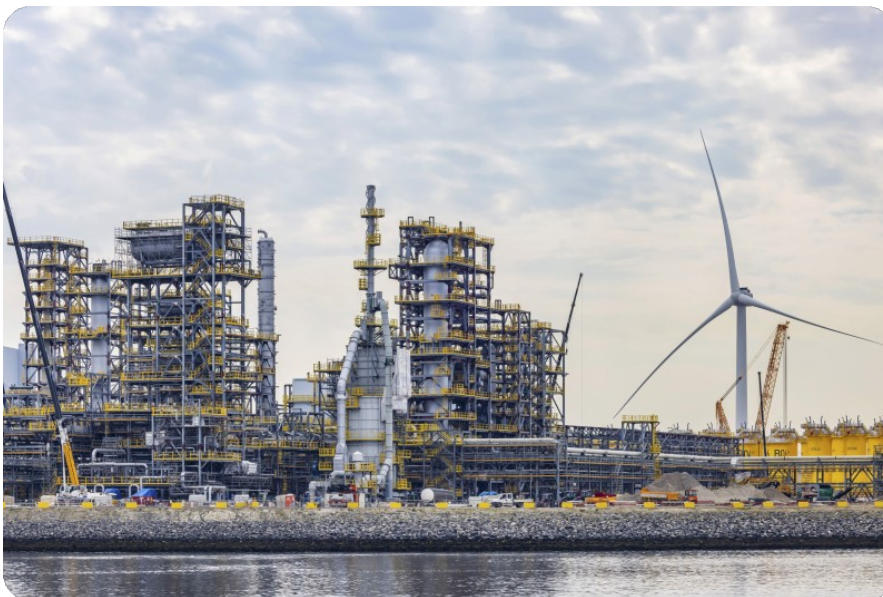
The Finnish company Neste is building a bio-refinery plant on artificial land in Rotterdam
