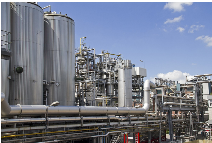
Chemical plant in Rotterdam, Netherlands
