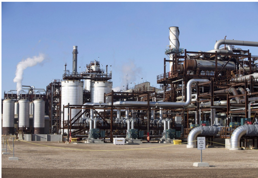
Quest carbon capture and storage facility in Fort Saskatchewan, Canada
