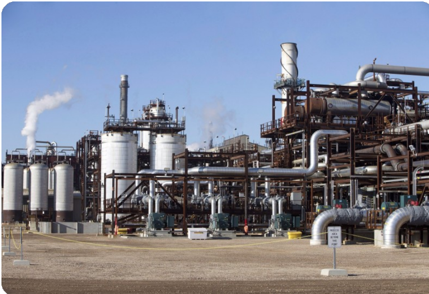
Quest carbon capture and storage facility in Fort Saskatchewan, Canada
