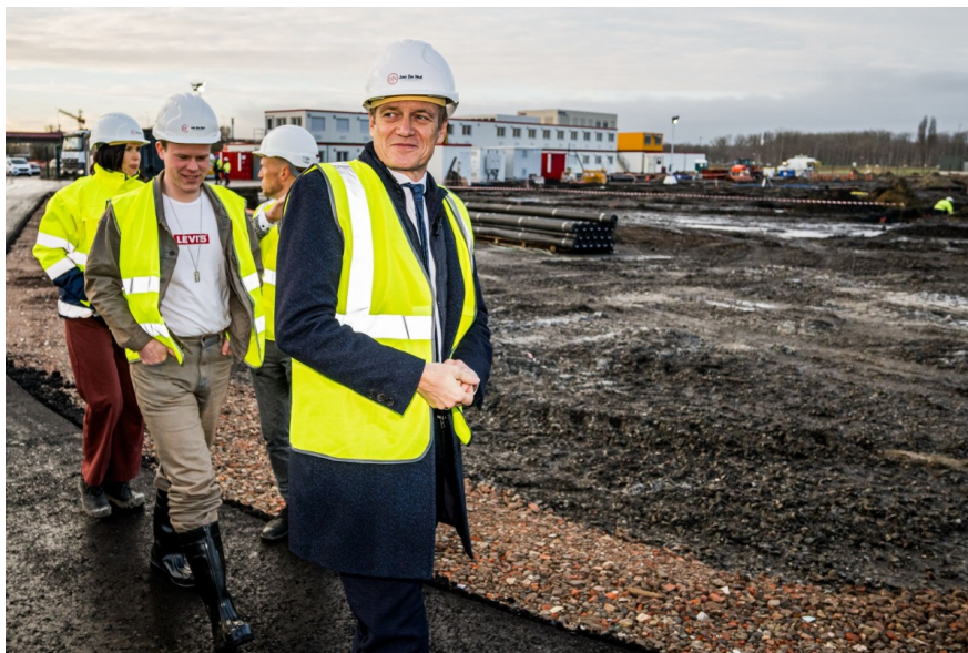
Belgium's Minister of Justice, Paul Van Tigchelt, visiting a new prison construction site in Antwerp
